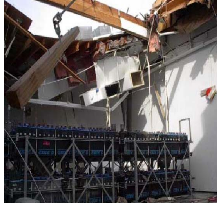
Photo of a battery room that exploded, resulting in massive property damage. Case study featured next page
